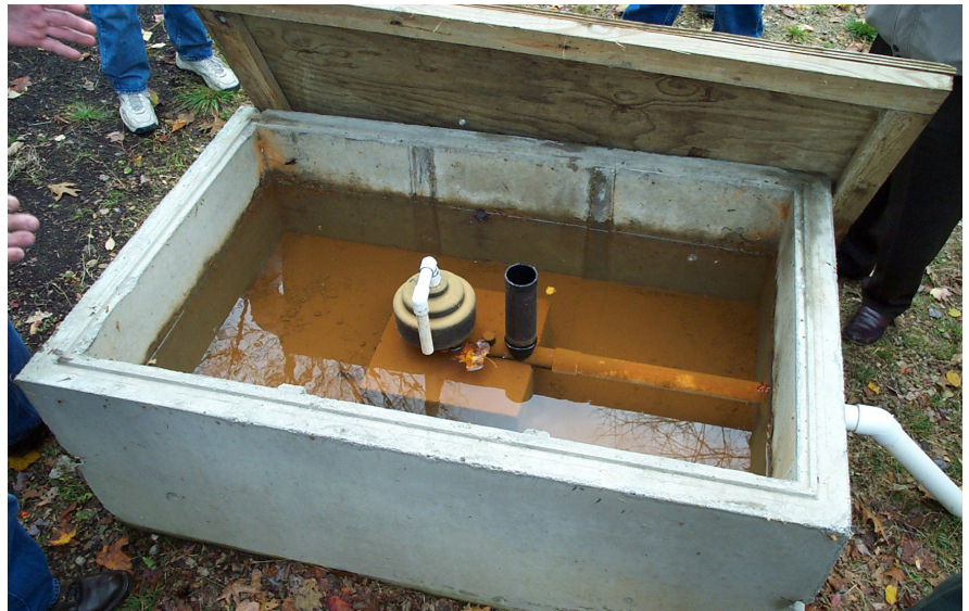
Figure 12: Siphon in dosing tank
