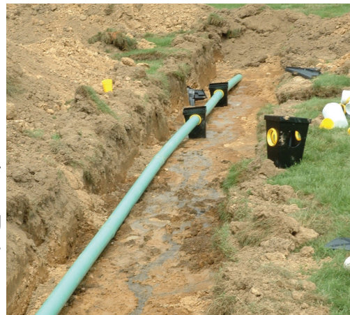
Figure 8: Distribution boxes on gravity manifold to equalize flow among drainfield lines.
